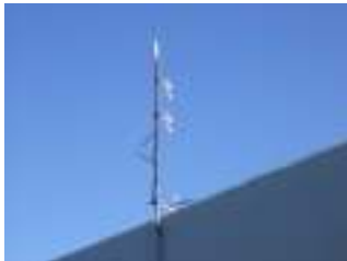
Antenna array on roof
